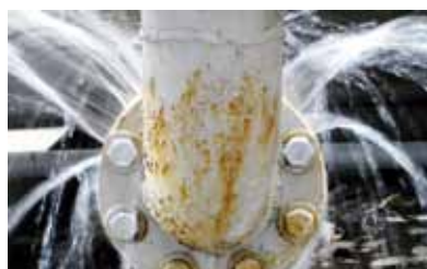
Pipeline & hydrant damage Extremely quick to set up in emergency situations
